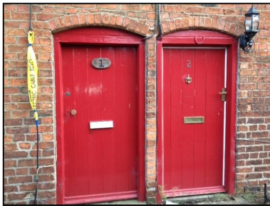
Fig.3 Timber panel doors at Blue Town
